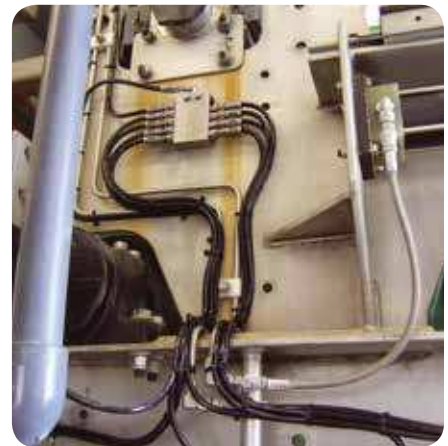
In this corrosive environment, a stainless steel Lincoln Quicklub system is lubricating and purging 32 points on a belt press in a wastewater plant.
