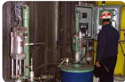
These Lincoln pumps deliver grease directly from a 400 lb. (181 kg) drum to 200 SL-V injectors located approximately 250 ft. (61 m) away in a steel mill.
