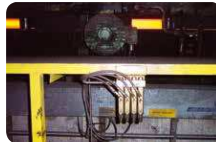
These SL-V injectors operate in a harsh steel mill environment that includes high heat and abrasive contamination. Purging the bearings, replacing the grease film frequently and increased safety are key benefits of this system.
