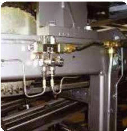
Stainless steel SL-32 grease injectors are used here to prevent corrosion from daily wash-down maintenance practices at this food plant.
